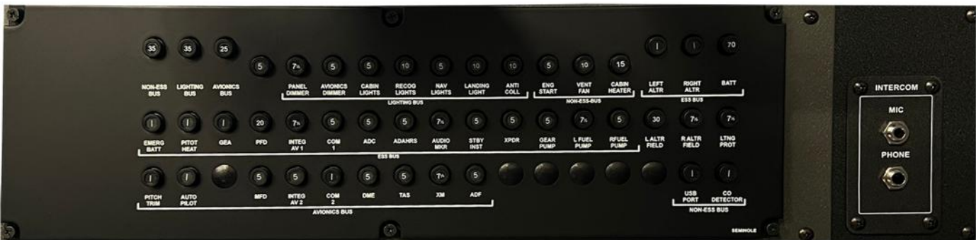
Seminole Circuit Breaker and Intercom
