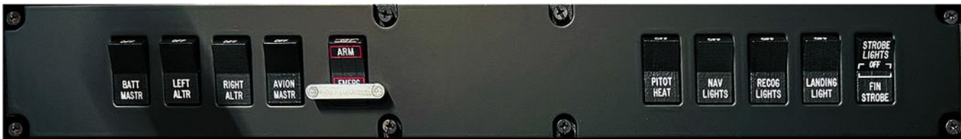
Seminole Battery Master and Lights Panel
