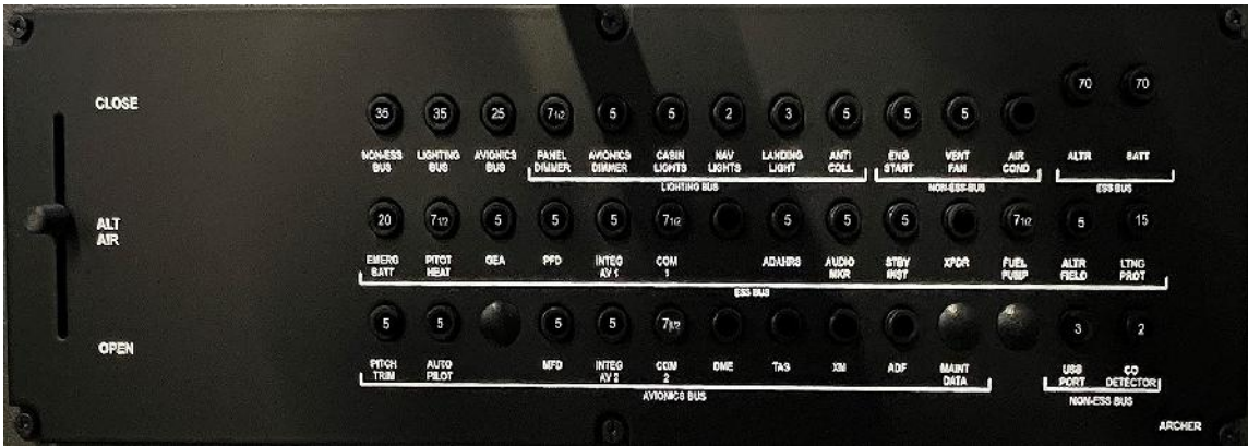
Archer Circuit Breaker Panel
